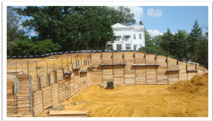
Figure 2: North Hall Soldier Beams, Lagging and Tiebacks Photo Taken By: Brandon Tezak
